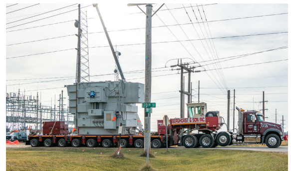
Contractors deliver the North Substation's new 161kV/69kV Auto Transformer
